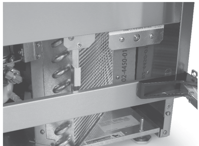
Condenser and Bin Thermostat
